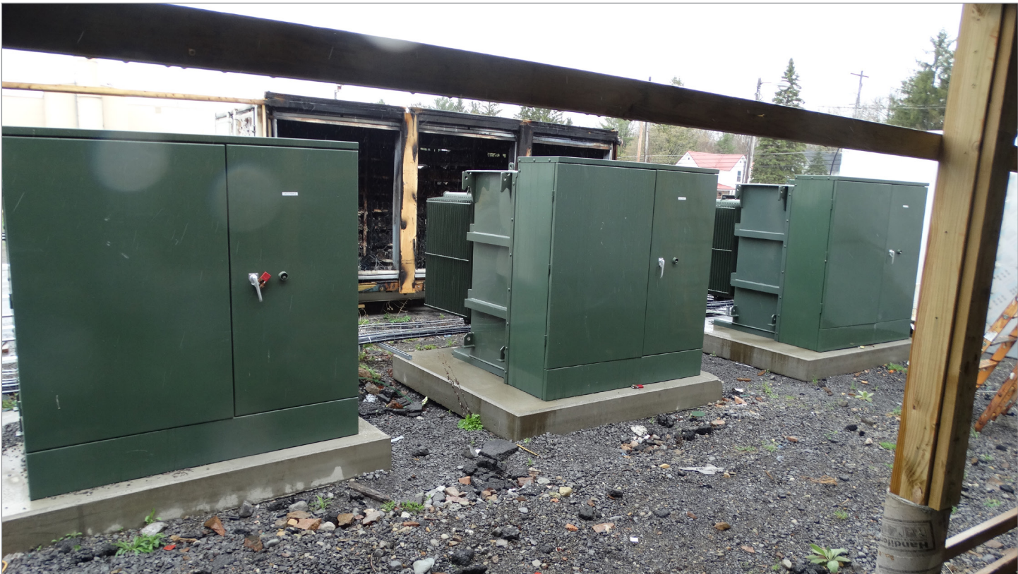
Pad mounted transformers in front of the shipping containers. Picture credit Envista Forensics.
