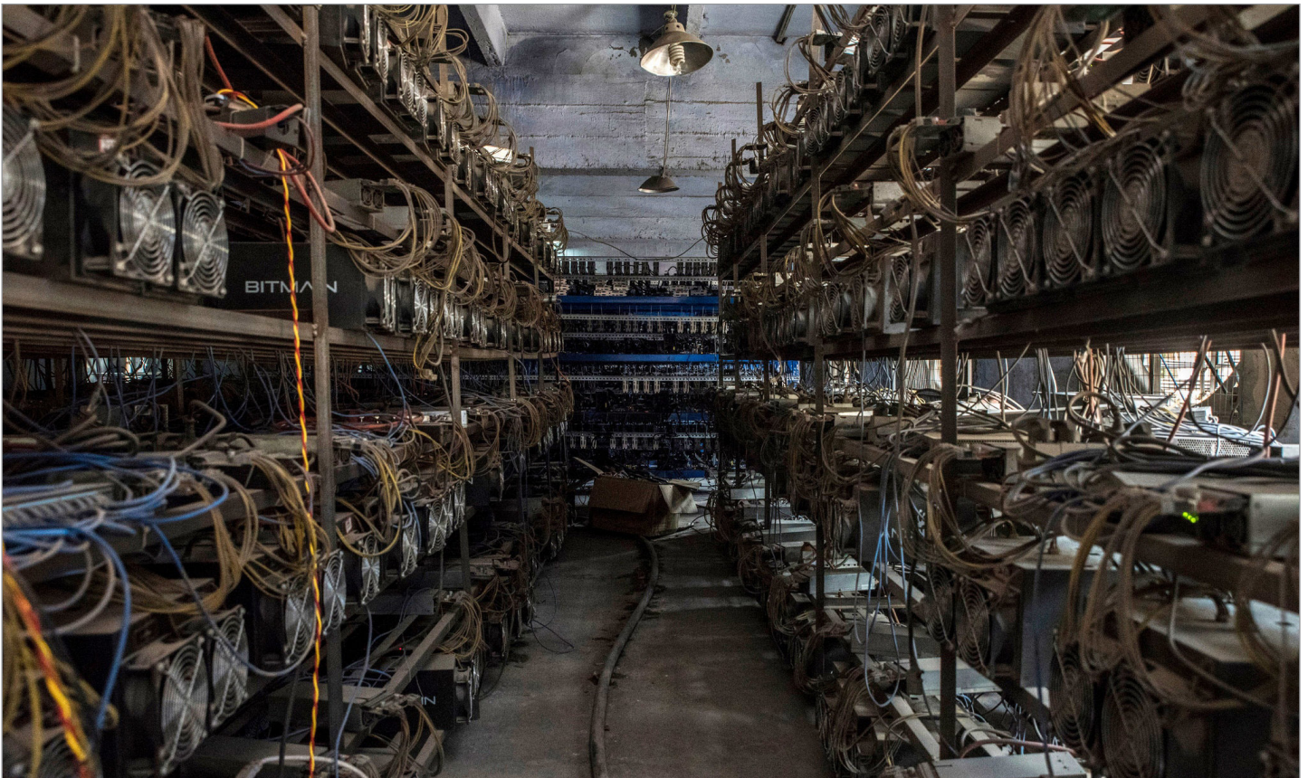
Mining servers in a repurposed building and the electrical feed into that building. Published with permission from Gilles Sabrie.
