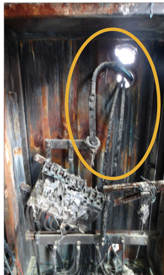
The electrical cable chafed wiring insulation in contact with the container. Picture credit Envista Forensics.
