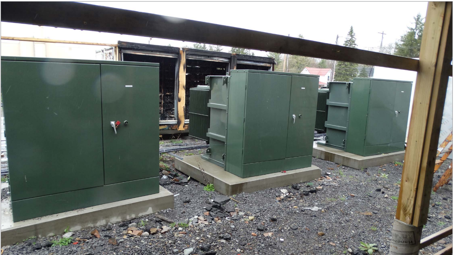
Pad mounted transformers in front of the shipping containers. Picture credit Envista Forensics.
